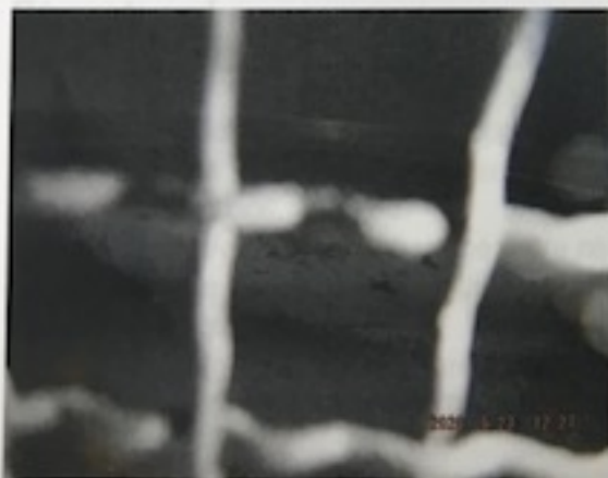
Roof vent screen
