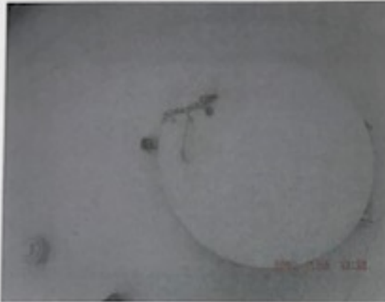
Roof access hatch locked
