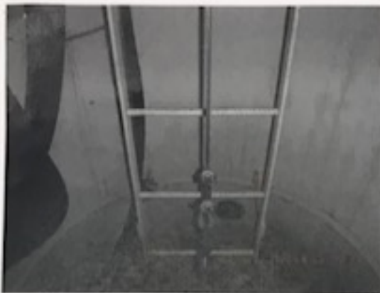
Safety climb cable
